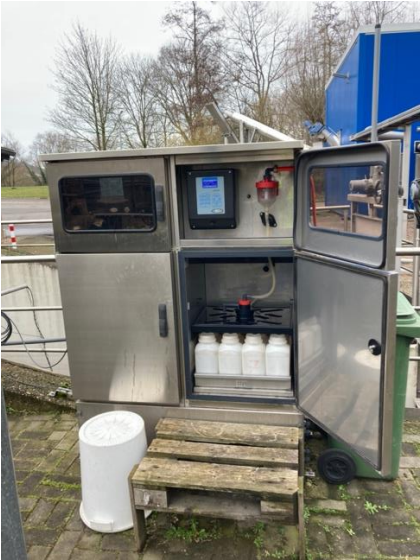
Figure 9 -Automated Sampling Device at the WWTP Aachen Soers (courtesy of F. Joerens, Wasserverband Eifel-Rur)
