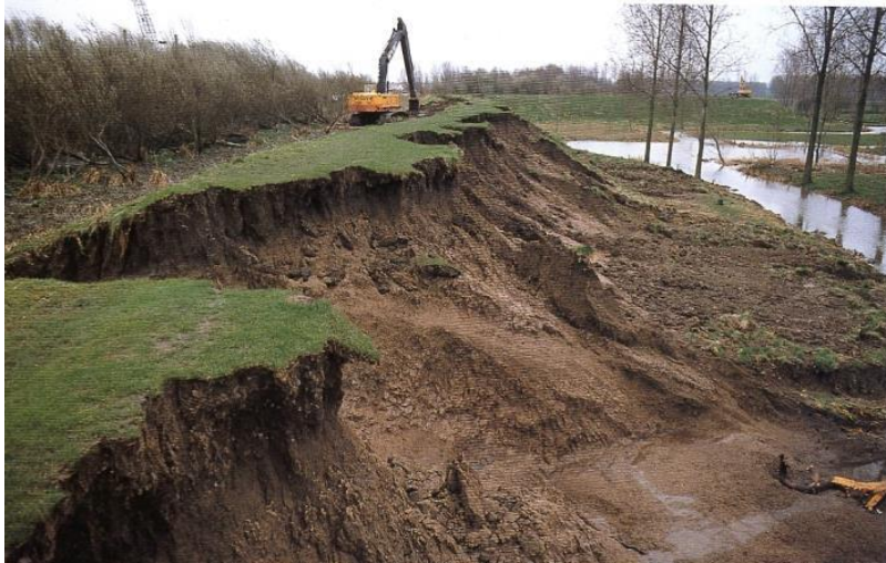
Figure B-10. Failure of the land-side slope along the Sea Scheldt in 1990 following overtopping (Source: A. Van Hoyweghen)
