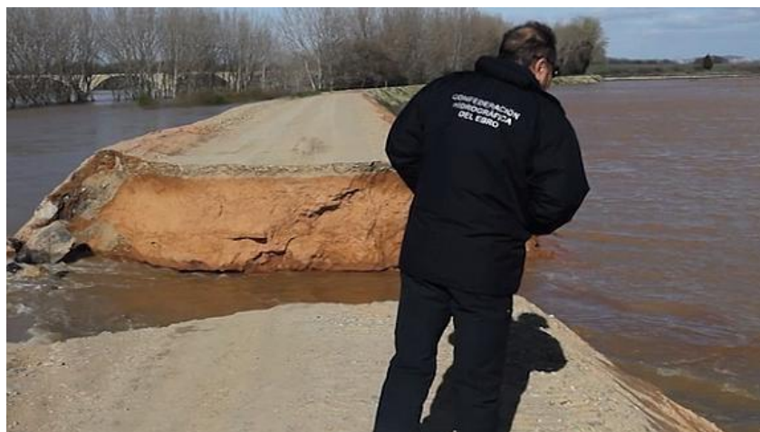
Figure ES-6. Example of partial failure in a levee due to an inadequate foundation.
