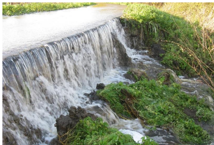
Figure B-14. Headcut formation following a low-head overflow event along the Durme in 2010 (Source: FHR)
