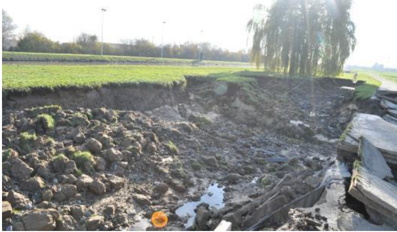
Figure B-12. Erosion following overflow along the canal Brussels (top left)– Charleroi in 2010 (Source: K. Van Eerdenbrugh)
