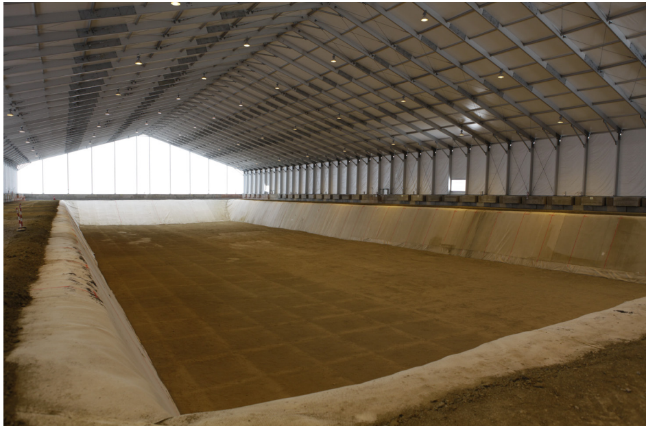
Image of the interior of the VLLW disposal vault at El Cabril.
