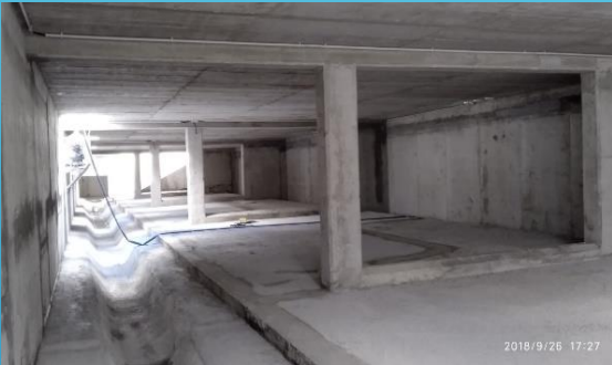
Interior tanque tormenta Puerto
