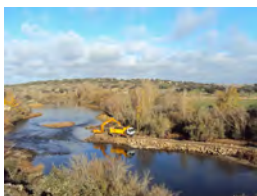
Improvement work on the fluvial system. Photograph taken from the Grupo Tragsa image bank.
