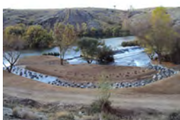
Improvement work on the fluvial system. Photograph taken from the Grupo Tragsa image bank.
