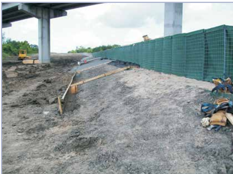
Figure 10.9 Temporary flood protection built to protect adjacent community during reconstruction of the existing flood protection (courtesy USACE)
