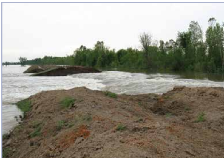
Figure 9.130 Earthfill embankment fuse plug after activation using explosives, Birdspoint-New Madrid floodway, Mississippi River (courtesy USACE Memphis District)
