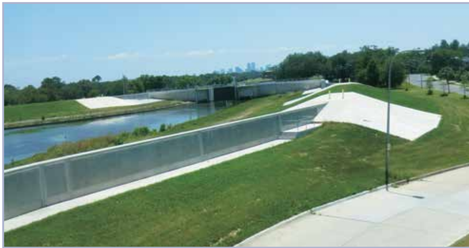
Figure 3.149 Transition in terms of the geometry of the levee: change in cross-section between a levee and a flood wall, New Orleans, Louisiana, USA (courtesy USACE)
