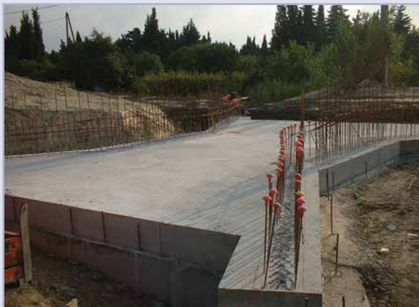
Figure 9.71 Concrete slab and beams cast directly into excavations, Aramon Levee, South of France (courtesy Thibaut Mallet)
