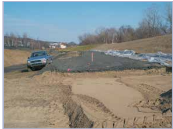
Figure 10.21 Spreading of material from borrow to determine appropriate lift thickness before compaction. Wooden lathes are used to control loose lift thickness (courtesy USACE)
