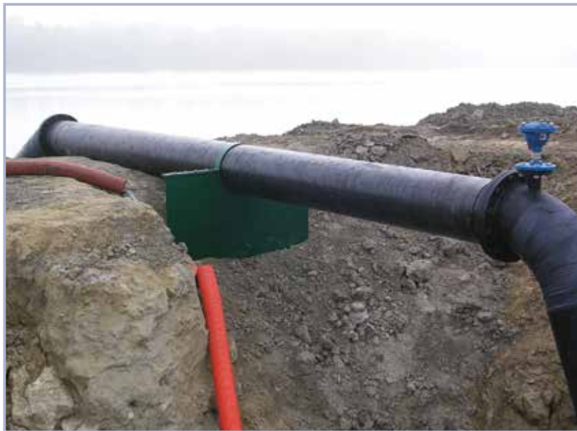
Figure 9.154 Pipe crossing of Rhône river in France (courtesy Symadrem)
