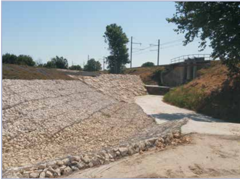
Figure 3.152 Transition between gabion basket and stone revetments, Rhone River, France (courtesy Jean Maurin)
