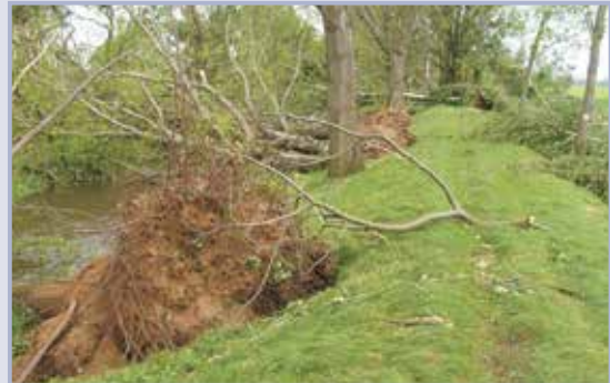
Figure 10.49 Reduced levee cross-section (and reduced stability) due to uprooted trees
