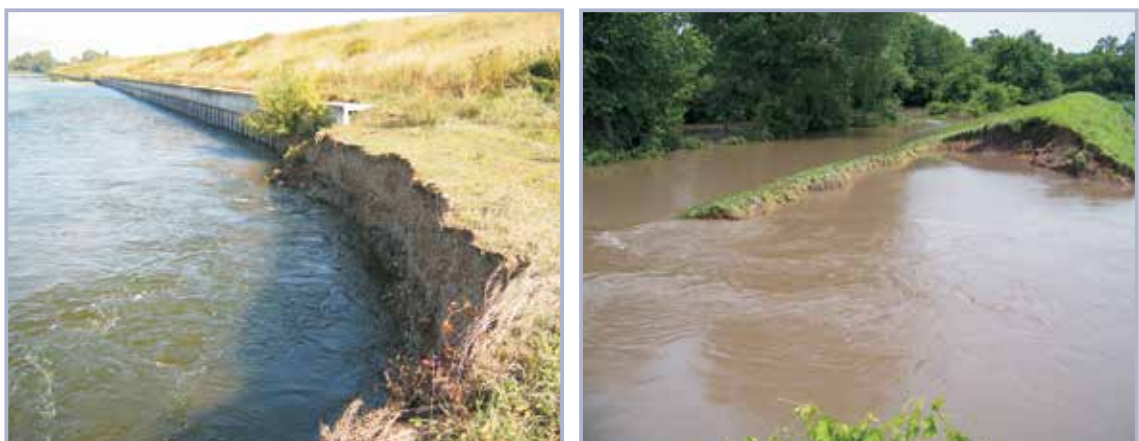
Figure 3.161 Breaches in Scott County, USA (courtesy USACE)
