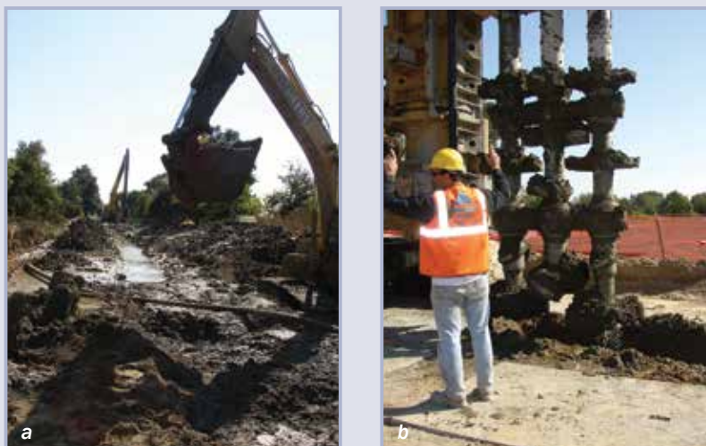
Figure 9.88 Seepage cut-off wall construction along levee centrelines, Sacramento, CA (courtesy Mike Wielputz, USACE)
