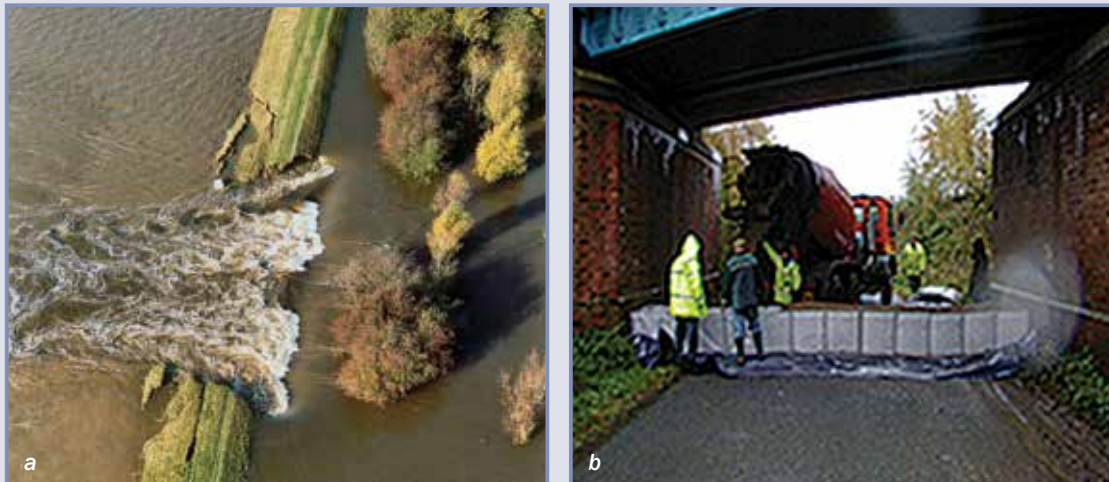
Figure 6.14 Levee breach in Gowdall (a) and temporary dam under construction on roadway under Drax railway line (b) (courtesy Environment Agency)
