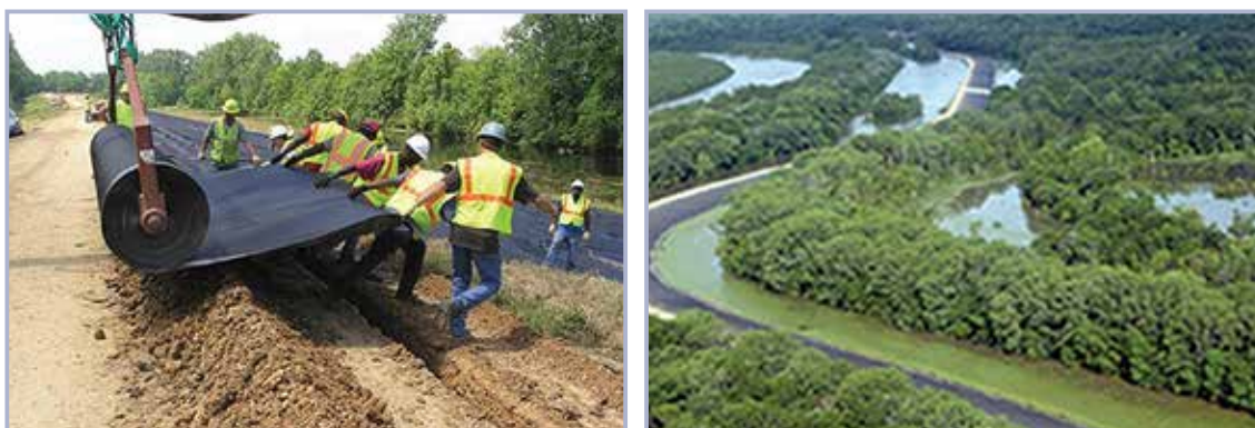
Figure 6.32 Use of plastic sheeting to prevent overtopping/overflow erosion, placing plastic sheeting on levee waterside (a) and finished placement (b) (courtesy USACE)
