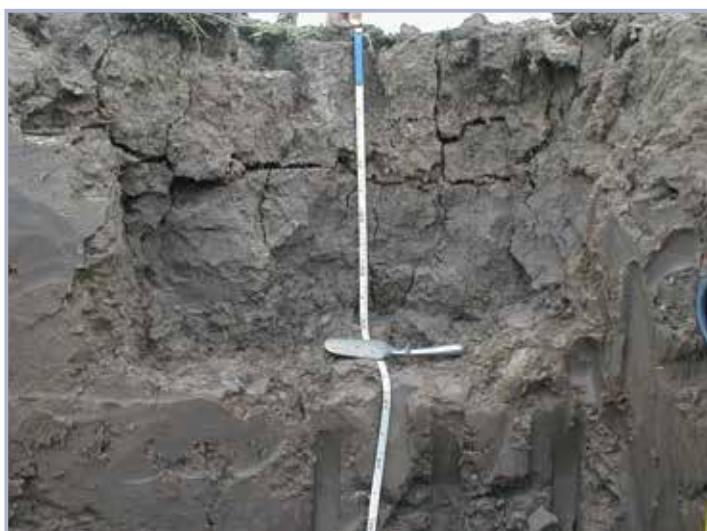
Figure 9.76 Desiccation cracking in levee at Thorgumbald (from Dyer et al. , 2009)
