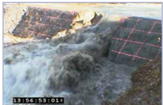
d Soil wasting – block failure on left face of breach 2s after failure of block breach (ie block has been removed)
