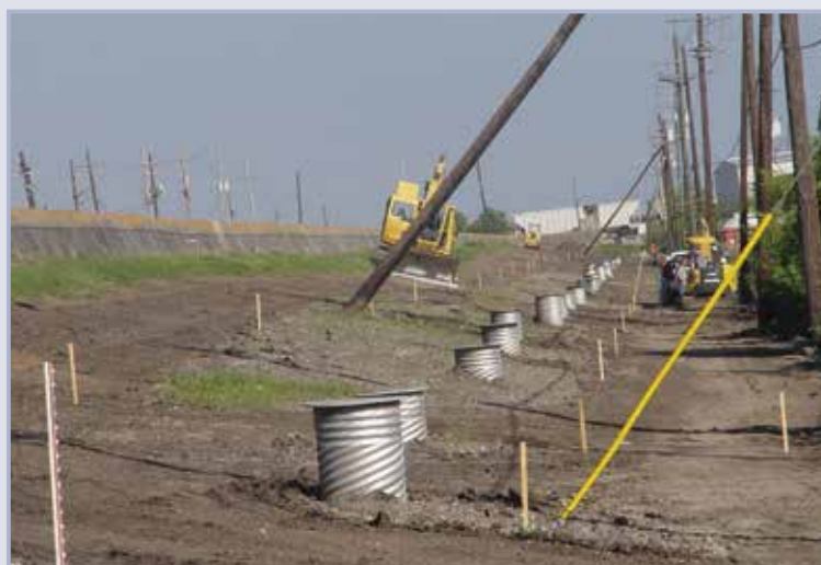
Figure 9.44 Completed relief wells at the landside toe connected to a buried collector pipe (looking north toward Lake Pontchartrain) (courtesy Richard Bird, URS)
