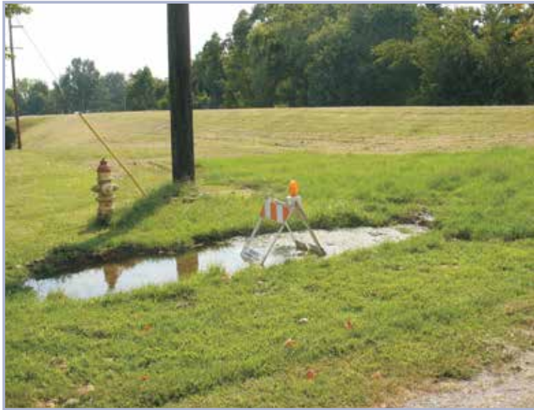
Figure 4.57 Evidence of water supply pipe leak – ponding of water at landside levee toe
