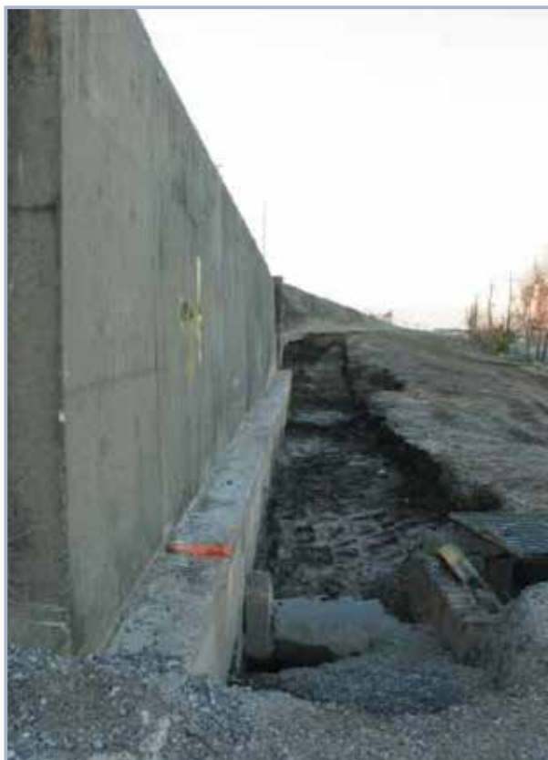
Figure 9.33 Scour trench at a T-wall on the east side of the IHNC following Hurricane Katrina, New Orleans, USA (courtesy USACE New Orleans District)
