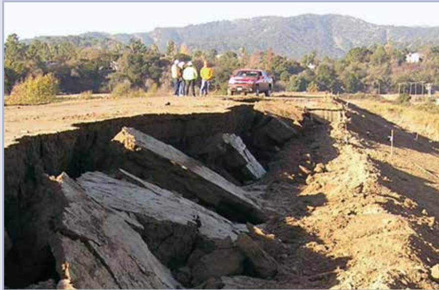
Figure 9.50 Levee failure at the end of construction, California, USA (courtesy Mary Perlea, USACE)
