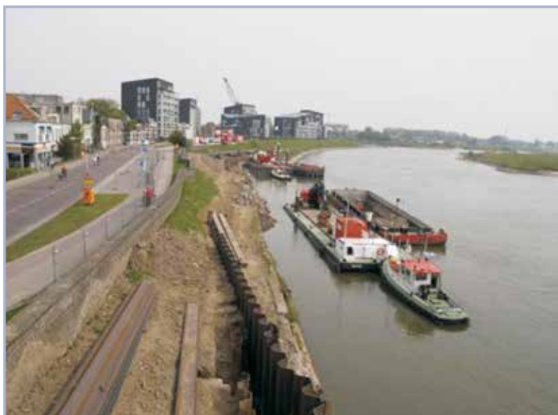
Figure 10.15 Transport of material over the river IJssel for the reconstruction of the quay Pothoofd in Deventer, the Netherlands (courtesy Harry Mols)
