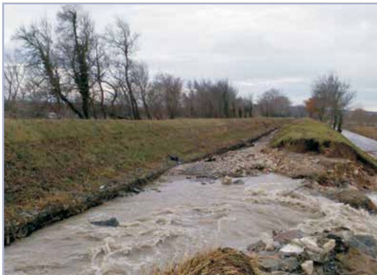
Figure 3.171 External erosion of the landward side (courtesy G Degoutte, Irstea)
