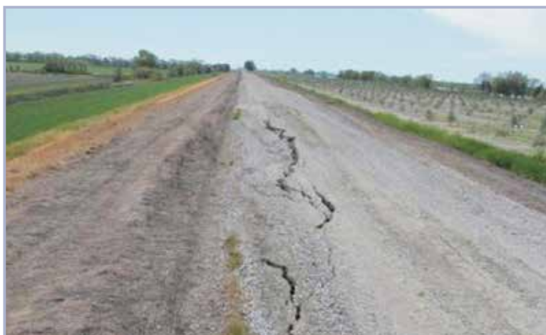
Figure 4.48 Structural crack running parallel to levee crest
