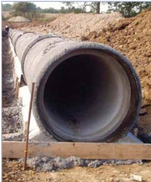
Figure 9.160 Pre-cast concrete pipe using bedding as support (from FEMA, 2009, courtesy FEMA and US Bureau of Reclamation)
