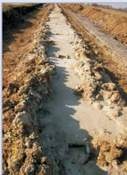
Figure 10.55 Soil cement cut-off wall after placing the reinforcement steel girders in certain spacing derived from stability calculations
