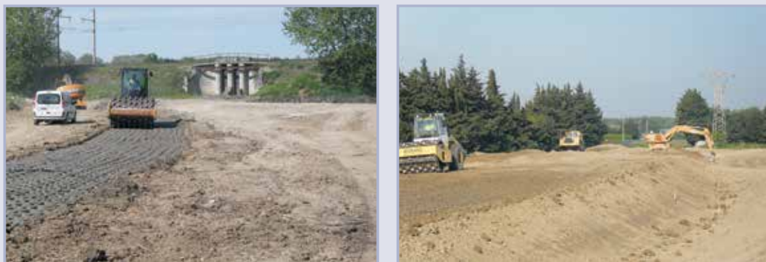
Figure 10.30 Backfill of the anchor trench and body of the levee with impervious material (courtesy EGIS)
