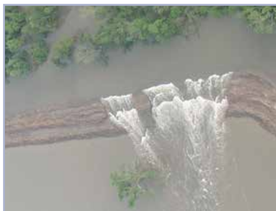
b Oblique view showing erosion of downstream levee slope following floodway operation plan
