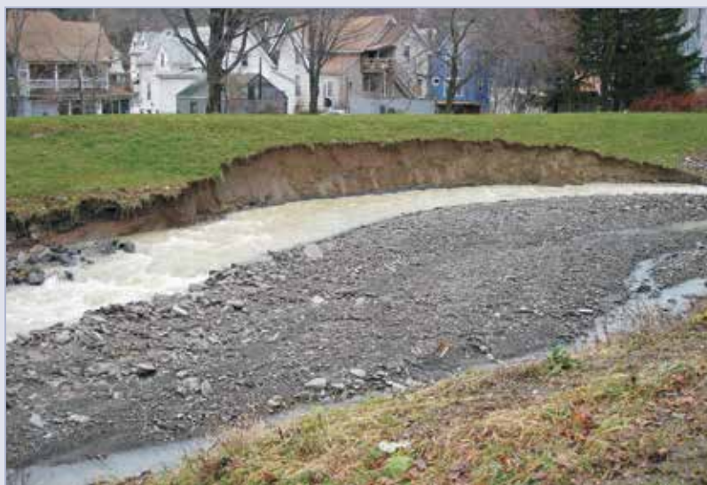
Figure 4.34 The effects of erosion on a levee slope at Park Creek, New York, USA
