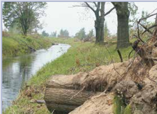
Figure 10.50 Cut trees to ensure the free flow in the river again. Stumps in the background on the right bank levee
