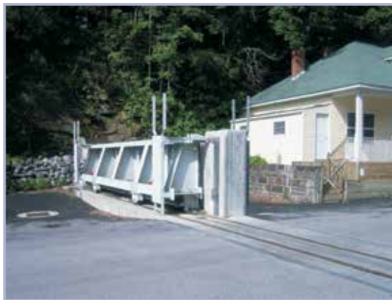
Figure 3.110 Slide closure (courtesy USACE)
