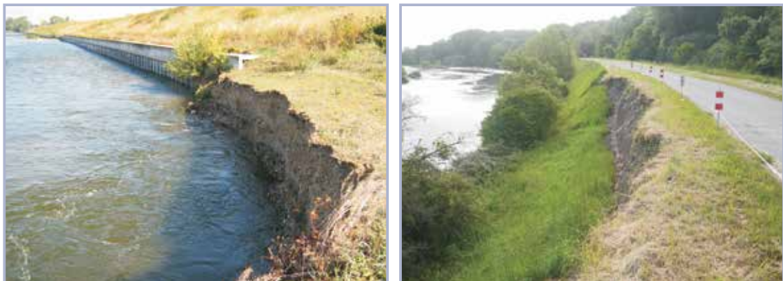
Figure 3.159 Erosion by river flow and instability due to undercutting toe (courtesy J-Y Hardy, DDT37 and E Durand, CETE NC)
