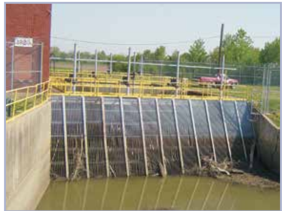
Figure 3.138 Pumping station trash rack (courtesy USACE)
