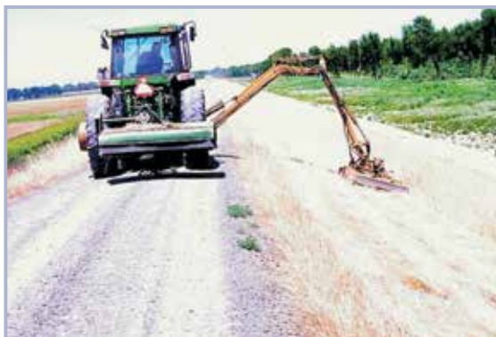
Figure 4.18 Mechanical mowing of grasses on California, USA, levee slope in dry season (courtesy California DWR)
