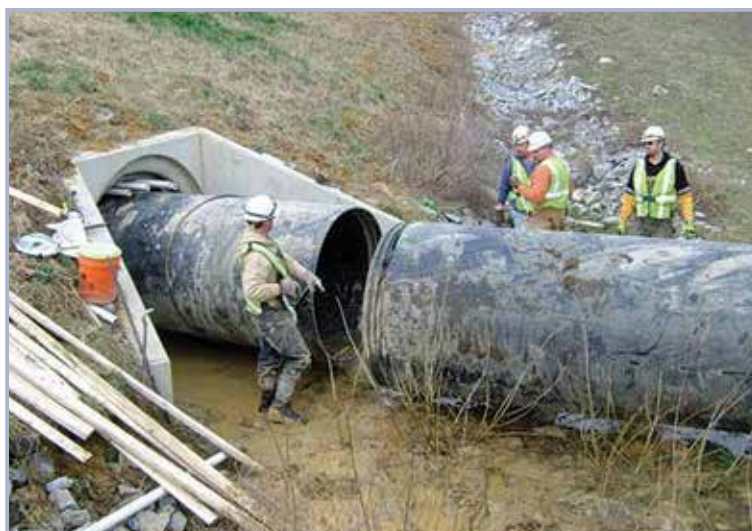
Figure 10.72 Typical installation of a segmental pipe liner on the New Albany Levee System in Indiana, USA (courtesy Christina Neutz)
