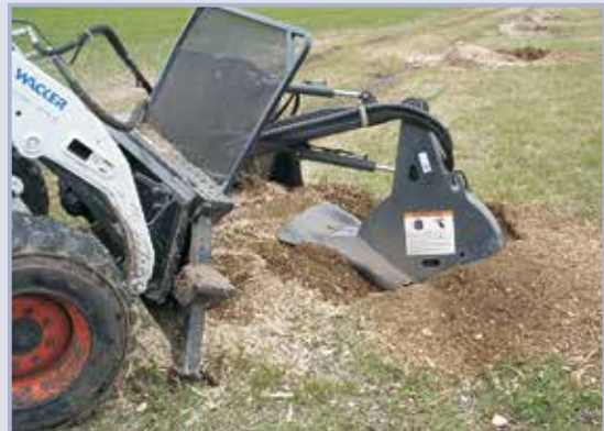
Figure 10.51 Milling and cutting the stumps and refilling the stump holes in and besides the levee
