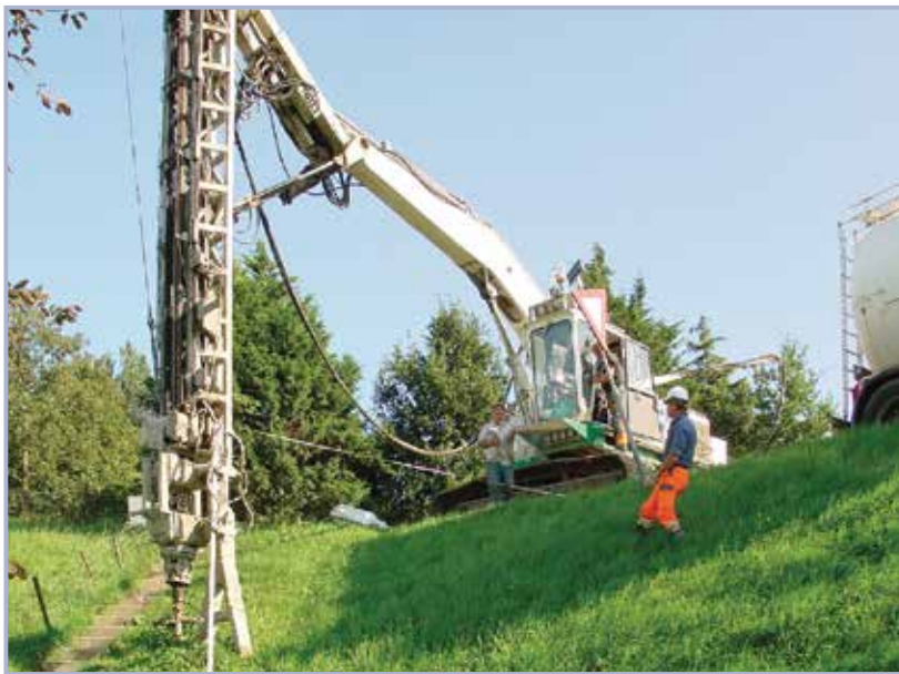
Figure 9.109 Deep soil mixing to facilitate levee raising (after de Kant and Wiggers, 2009, courtesy Keller Ltd and Royal HaskoningDHV)
