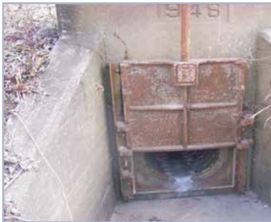
Figure 3.117 Slide gate (courtesy USACE)
