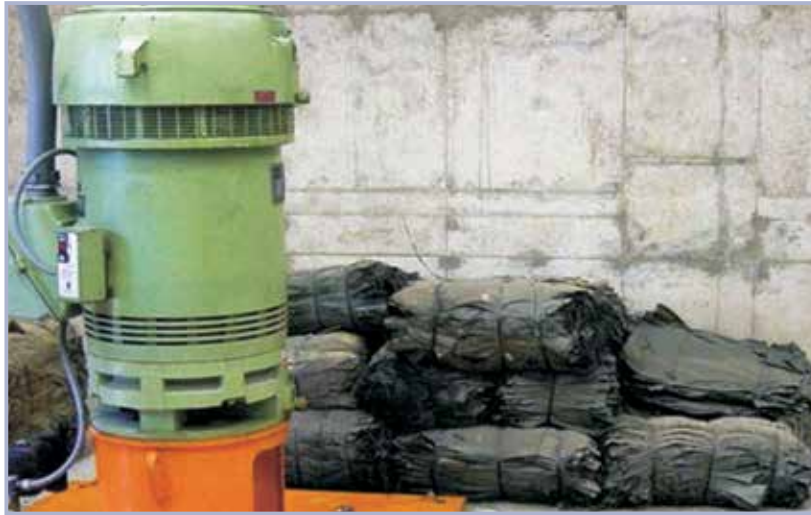
Figure 6.18 Sandbag storage at a levee pumping station (courtesy USACE)
