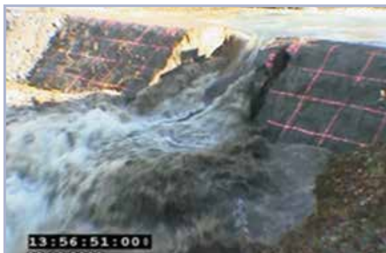
c Soil wasting – block failure on left face of breach
