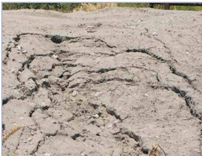
Figure 4.44 Tension cracks in the levee slope (indicating that slumping is occurring)
