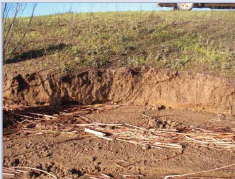
Figure 9.56 Waterside slope failure after rapid draw-down, Sacramento River levee, California (courtesy Mary Perlea, USACE)
