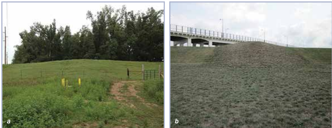
Figure 9.152 Utility pipes crossing up and over Paducah Kentucky Levee System (a) and the Cincinnati Ohio Levee System (b) (courtesy City of Paducah and Metropolitan Sewer District).
