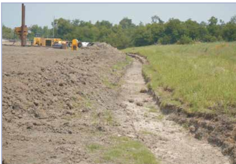
Figure 10.11 Temporary drainage ditch dug to ensure proper drainage during construction (courtesy USACE)
