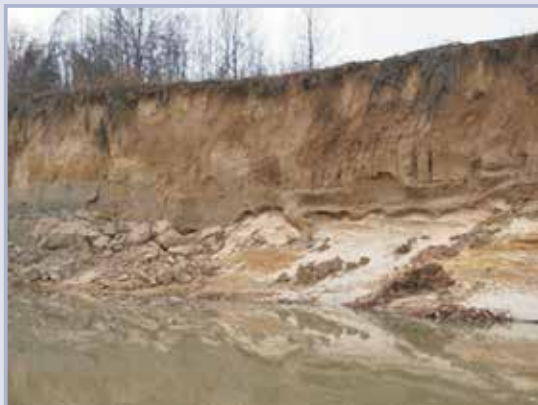
Figure 7.6 Moderate to severe bank erosion, bank height is approximately 10 m (courtesy Andy Gaines, USACE)
