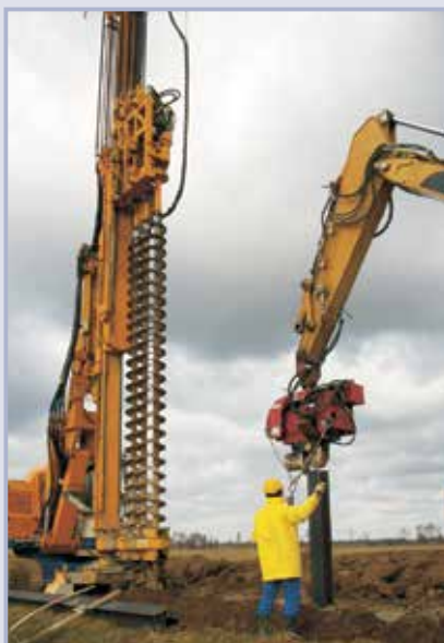
Figure 10.54 Mixed in place technique (MIP) was used along a 6950 m long reach. On the left: triple auger to break up the soil and to mix in the binder suspension. On the right: placement of steel girders into the still fresh soil-cement mixture
