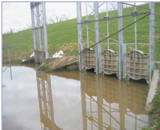
Figure 3.119 Slide gate mounted to headwall (courtesy USACE)
