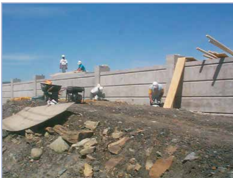
Figure 10.69 Flood wall riverside (courtesy USACE)
