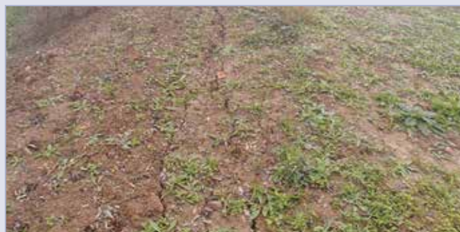
Figure 4.38 Cracks in the levee crest such as these should be taken seriously. Preventive action such as the installation of an adequate drainage system is recommended (courtesy Y Nedelec)
