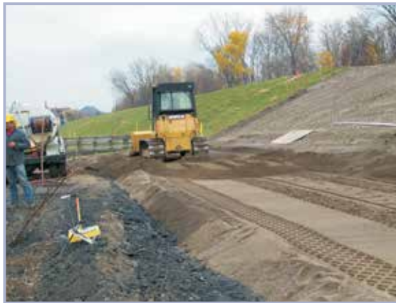
Figure 10.20 Spreading of material into uniform loose lift thickness before compaction (courtesy USACE)
