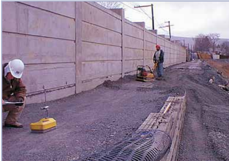
Figure 10.70 Concrete flood wall (background) and mechanically stabilised earth wall (foreground) (courtesy USACE)
