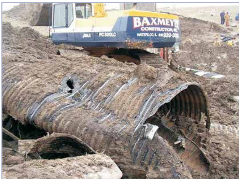
Figure 3.113 Culvert failure in Missouri (courtesy USACE)
