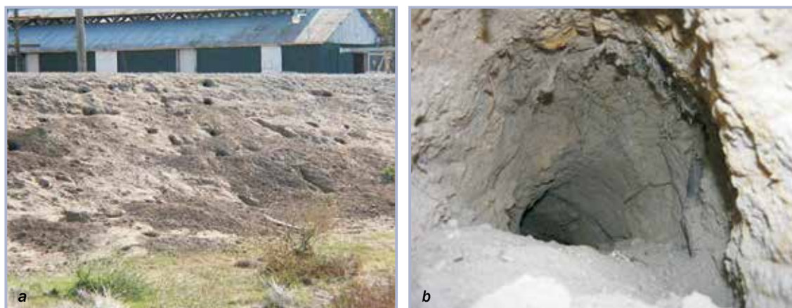
Figure 4.30 Holes caused by animal burrowing, (a) greater than five holes in a 10 m stretch of levee, and (b) a single hole larger than 15 cm in diameter
