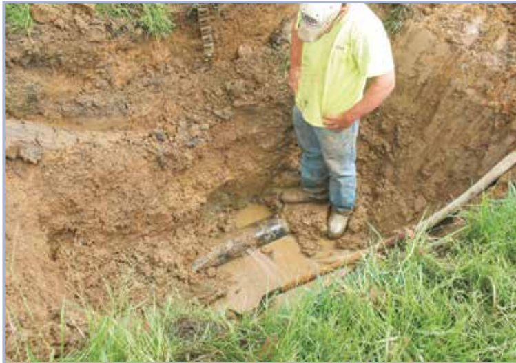
Figure 4.58 Open cut repair of leaking water supply pipe that penetrated a levee (least desirable repair technique due to cost and disturbance to the levee prism)
