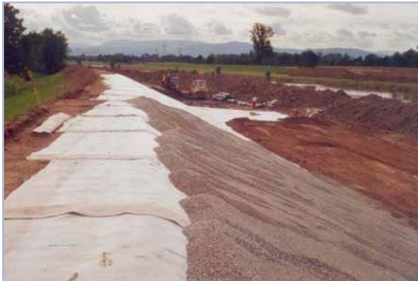
Figure 9.84 Covering geosynthetic clay liners with locally available gravel to ward off burrowing animals (Heerten and Werth, 2006)
