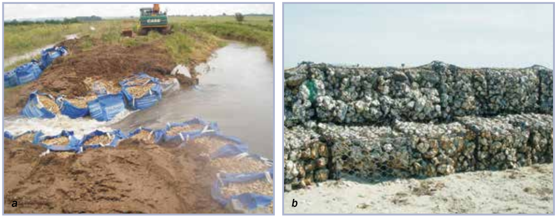
Figure 6.44 Response to levee breach, limiting breach growth using big bags (a) and gabions (b) (courtesy Environment Agency)
