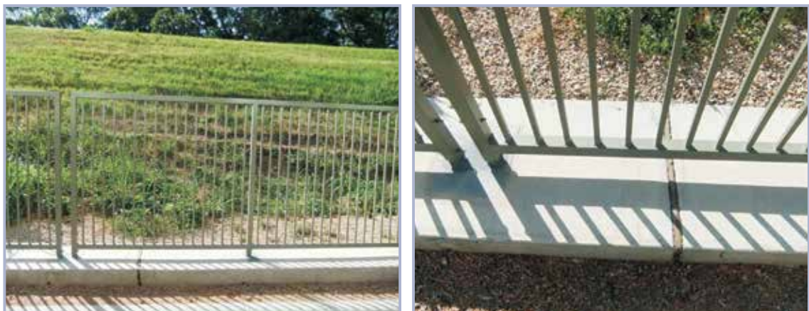
Figure 3.21 Aesthetic fencing along levee toe (courtesy Les Perrin)
