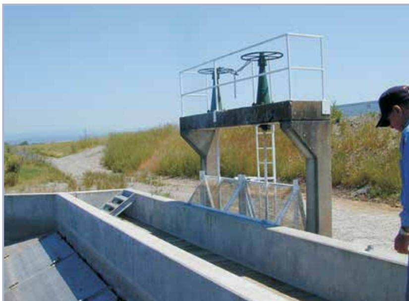
Figure 4.8 Pipe encroachment passing through the levee, Butte Creek levee, California, USA
