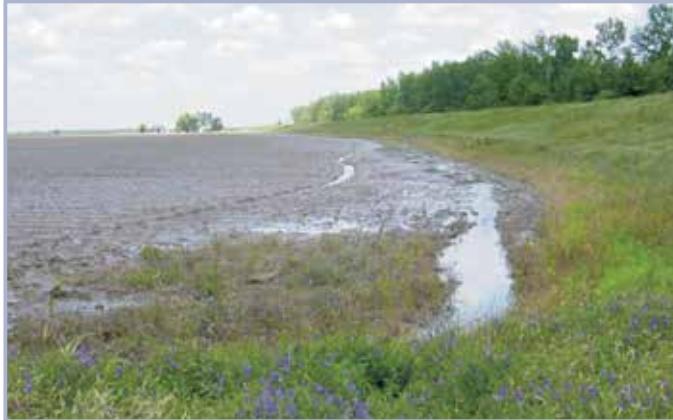
Figure 4.41 Seepage at the landside levee toe
