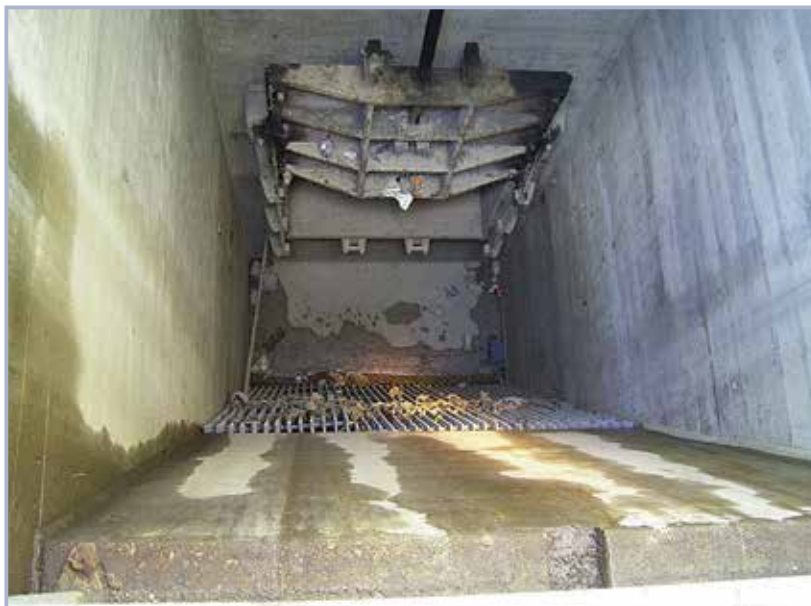
Figure 3.121 Sluice gate within a gatewell structure (courtesy Covington Kentucky Levee System, Louisville District, USACE)
