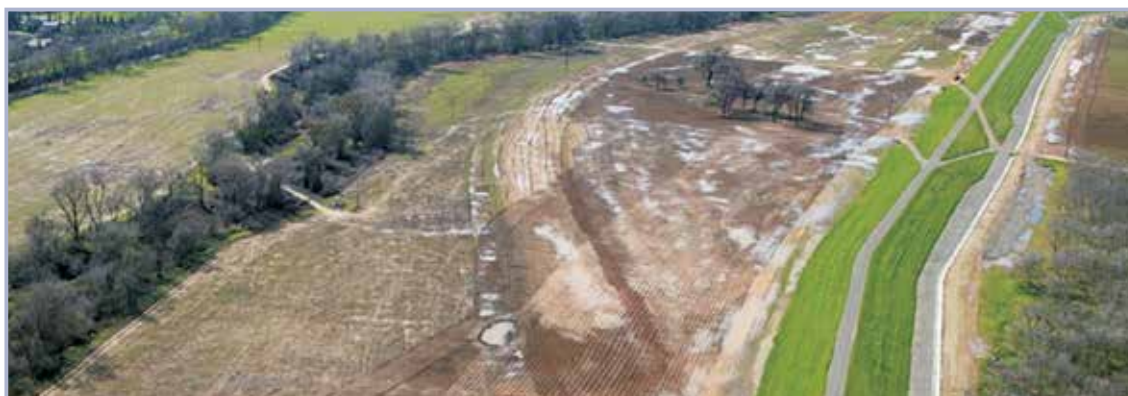
Figure 4.16 New grass cover growing on recently constructed Bear River setback levee, California, USA (courtesy California DWR)
