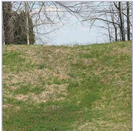
Figure 5.39 Depression in the levee crown directly above a deteriorated corrugated metal pipe (courtesy Louisville District, USACE)
