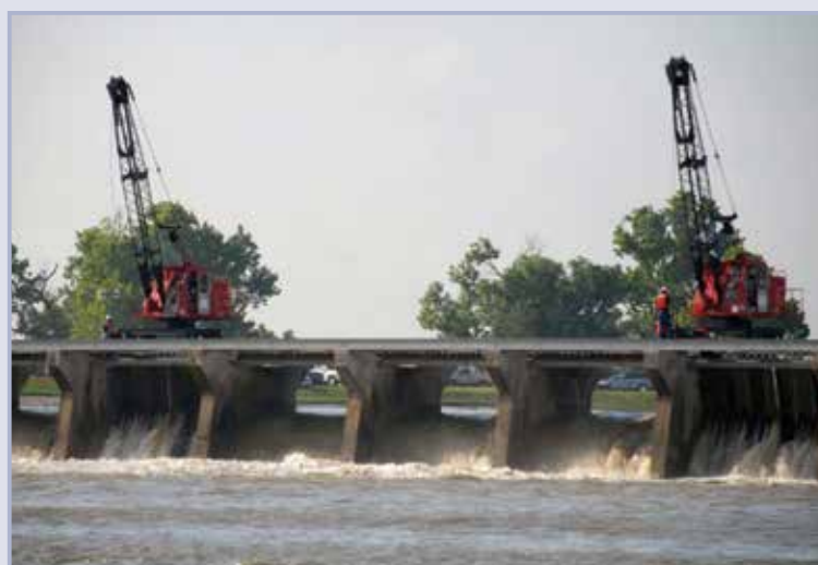
Figure 9.134 Cranes removing needle timbers to open spillway, Bonnet Carré control structure (courtesy USACE New Orleans District Archives)
