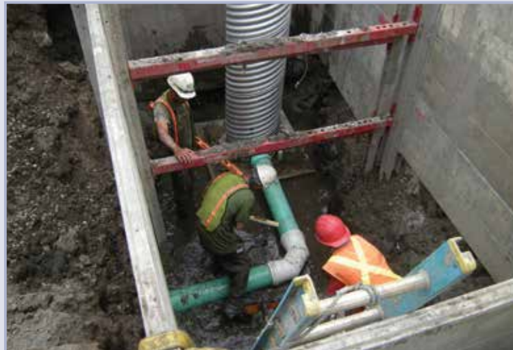
Figure 9.43 Connecting new relief well to buried collector pipe (courtesy Richard Bird, URS)
