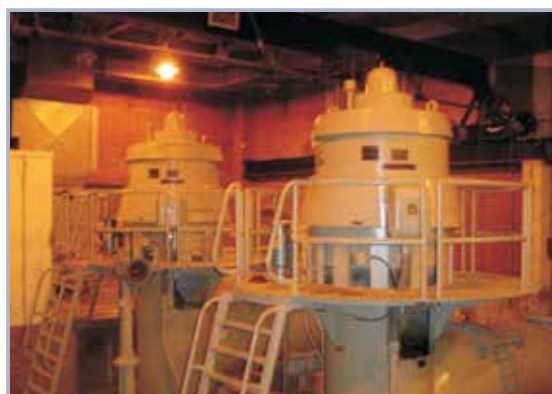
Figure 3.140 Interior of a pumping station (courtesy St Louis District, USACE)
