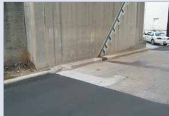
Figure 4.60 Restored concrete sill and new asphalt over where gas line entered the sill
