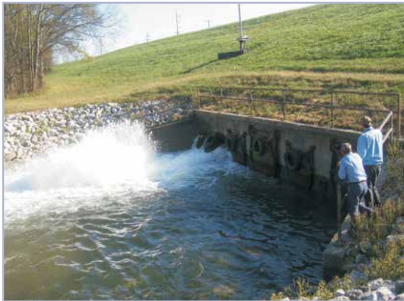
Figure 3.115 Release from pumping station discharge pipe (courtesy Paducah Kentucky Levee System, Louisville District, USACE)
