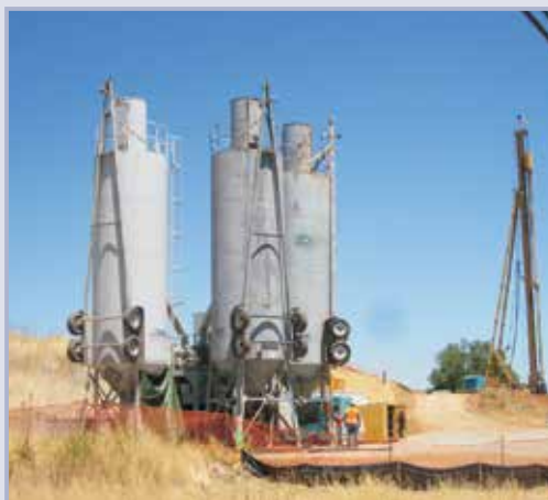
Figure 10.19 Seepage mitigation with deep soil mixing in Marysville, CA, USA (courtesy USACE)
