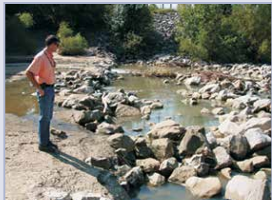
Figure 7.7 Stream bed instability and use of armour to stabilise stream profile (courtesy Andy Gaines, USACE)
