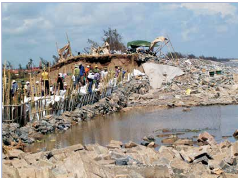
Figure 6.45 Emergency repair of coastal levee Nam Dinh, Vietnam after Storm no.7 (2005) (courtesy VNICZM project, Nam Dinh pilot office)
