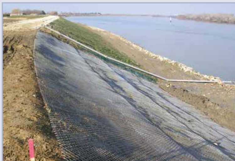
Figure 9.82 Wildlife protection mesh incorporated into levee improvement works at Arles, France (courtesy SYMADREM and EGISeau)
