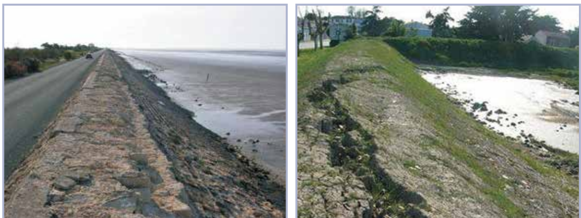
Figure 3.157 Wave damage and rotational sliding (courtesy R Tourment, Irstea)
