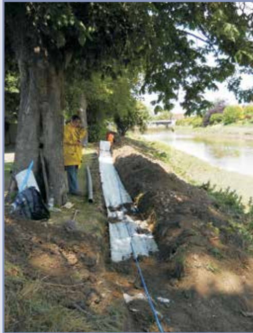
Figure 6.4 Fibre optic cable in geotextile fabric being laid in levee to measure ground strains at a pilot site (courtesy Victoria Bennett, RPI)
