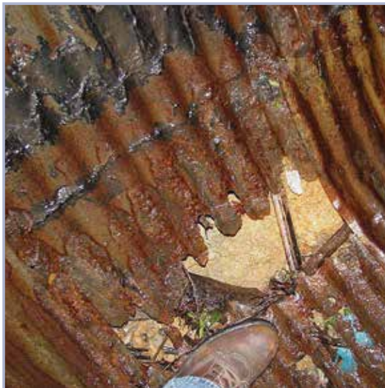
Figure 5.38 Complete section loss in the bottom of a corrugated metal pipe (courtesy Louisville District, USACE)
