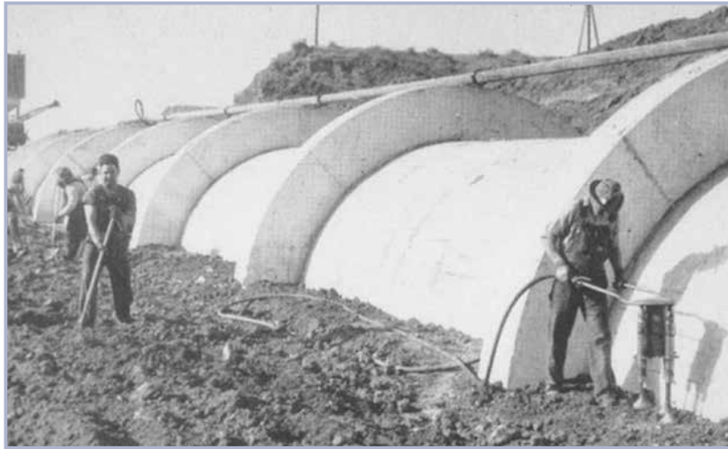
Figure 9.159 Difficulties of compacting around anti-seepage collars (from FEMA, 2009, courtesy FEMA and US Bureau of Reclamation)
