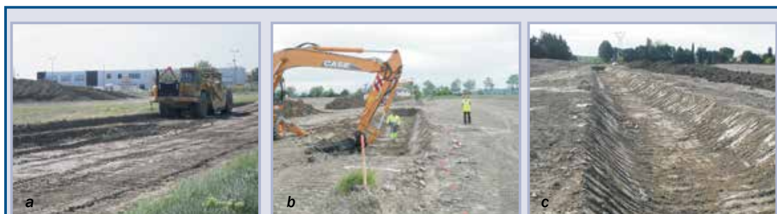
Figure 10.29 Preparation of site between agricultural parcels (a), excavation of anchor trench (b), develop localised drainage (c) (courtesy EGIS)
