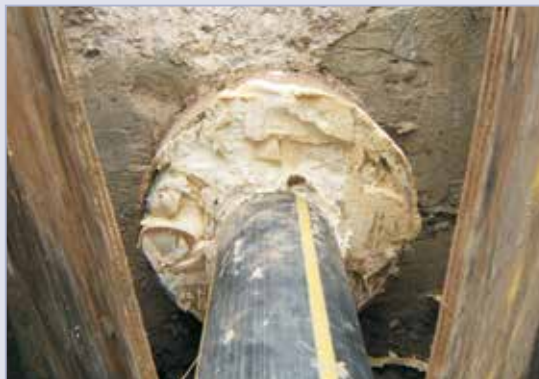
Figure 4.59 Polyethylene (PE) high pressure gas line within steel casing (encased within the concrete closure sill). Annular space filled with an expanding foam
