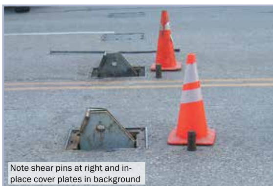
Figure 4.54 Truss shoes in their cast steel anchorages
