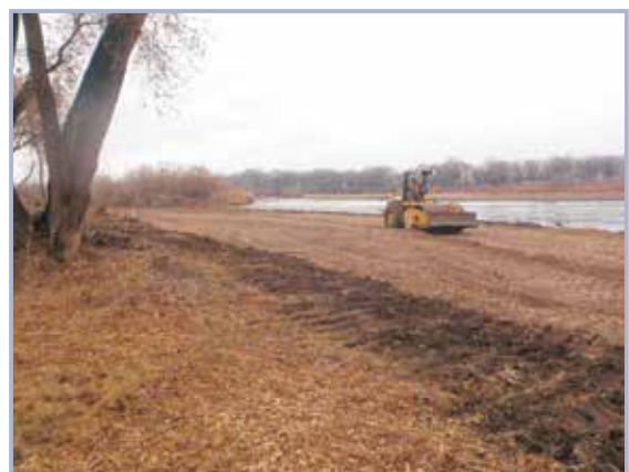
Figure 10.23 Compacting impervious fill using a pad foot roller to determine acceptable lift thickness and number of passes to achieve required density (courtesy USACE)
