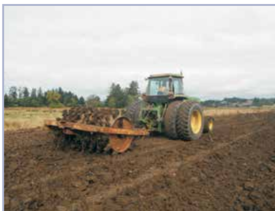
Figure 10.22 Compaction of material with a towed tamping roller to determine acceptable range of moisture contents to achieve specified density (courtesy USACE)
