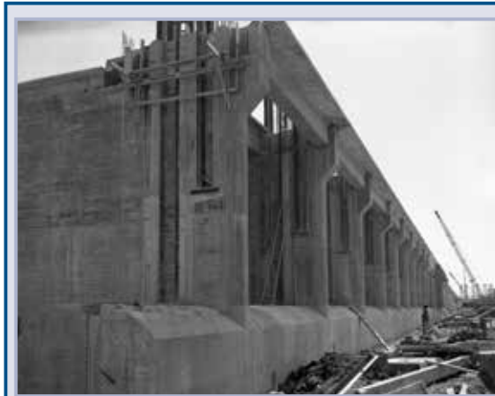
Figure 9.143 Construction of Morganza control structure, Mississippi River (courtesy USACE New Orleans District Archives)
