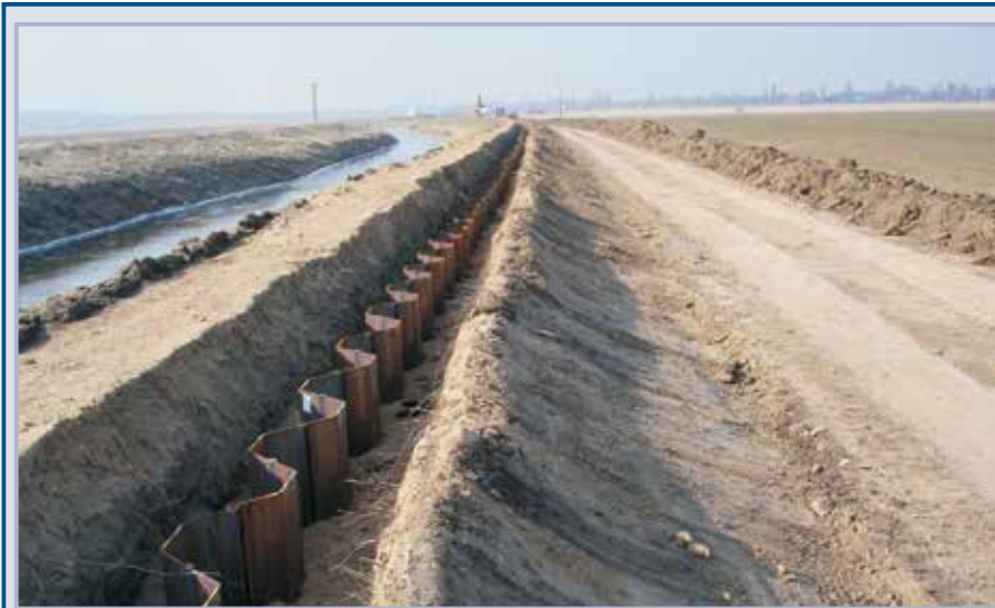
Figure 10.56 A 6250 m long sheet piling section of the levee. The sheet piling ends as well as the soil cement diaphragm walls below the final levee crest so that it will not be visible after completion of the refurbishment
