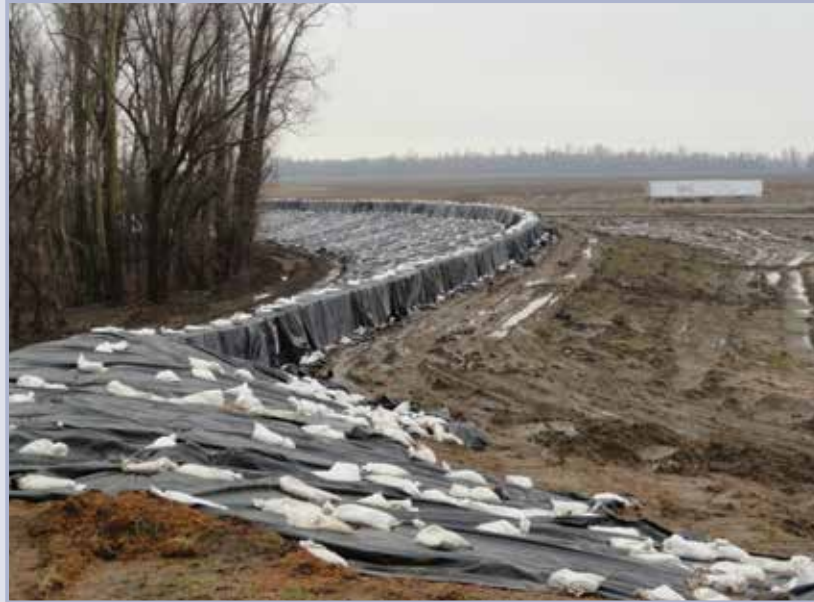
Figure 9.31 Polyethylene sheeting placed over newly constructed levee to provide temporary erosion protection (courtesy USACE Memphis District)
