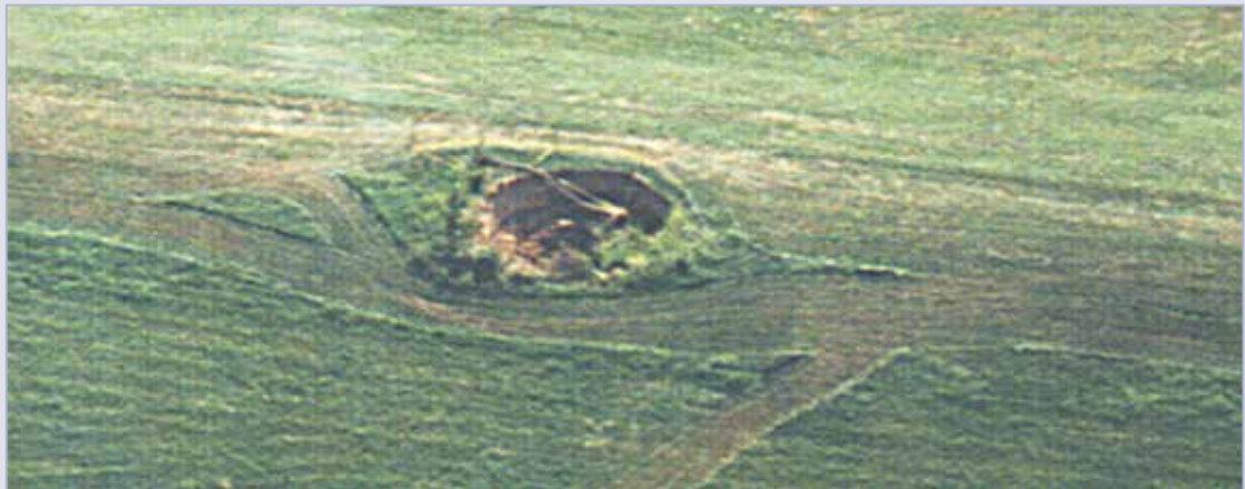
Figure 4.56 Sinkhole created when two 1.8 m diameter corrugated metal pipes collapsed under a levee in Indiana, USA
