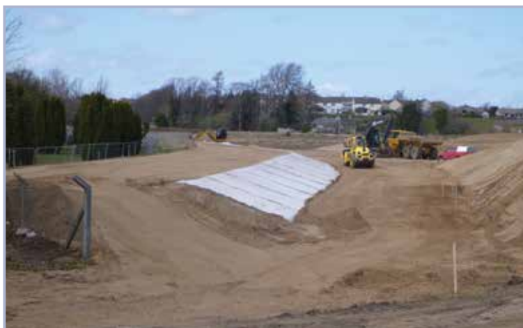
Figure 9.106 Geosynthetic clay liner being incorporated into a sand levee in Elgin, Scotland (courtesy Mark Donoghue, Royal HaskoningDHV and Moray Flood Alleviation)
