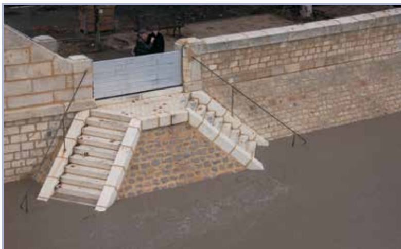
Figure 3.14 Floodgate access (courtesy Symadrem)
