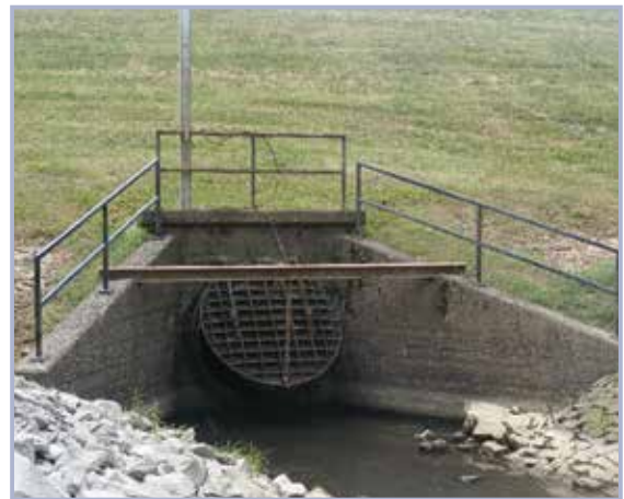
Figure 3.118 Flap gate (courtesy USACE)
