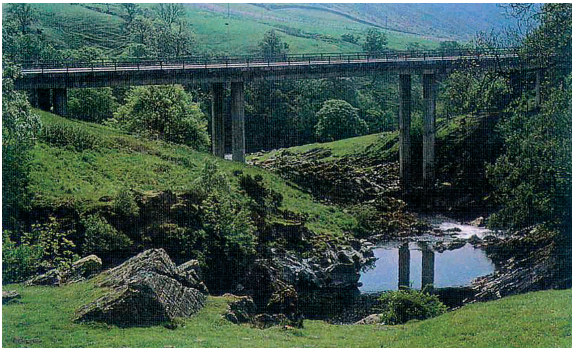
Figure 7.35 - This viaduct in northern England leaves the river valley intact. (Photo by Highways Agency, UK)
