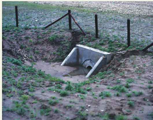
Figure 7.57 - This tunnel in the Netherlands has been filled with sand and water. The lesson learned from this example is to construct a tunnel above the ground water level and to build stable slopes around the entrances. (Photo by H. Bekker)
