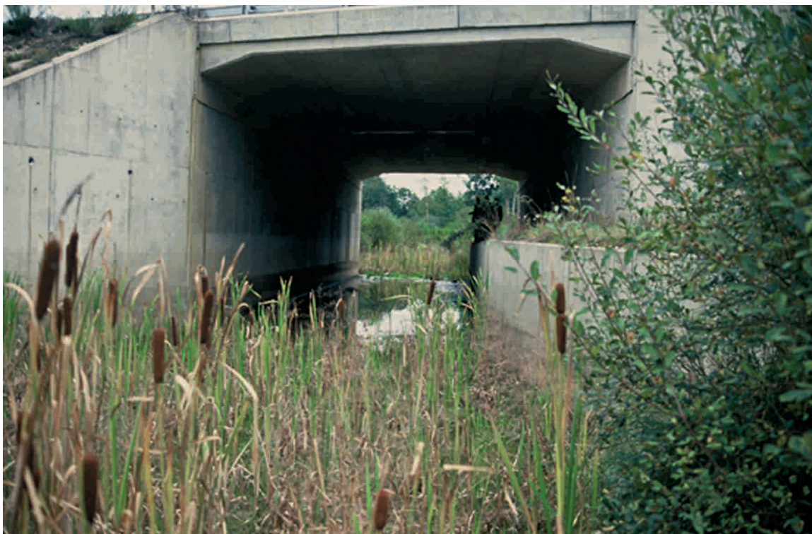
Figure 7.51 - The main purpose of this underpass at the A10 in France is water management in a wetland. The dimensions and the integrated ledge allow movement of small and medium-sized mammals. (Photo by H. Bekker)
